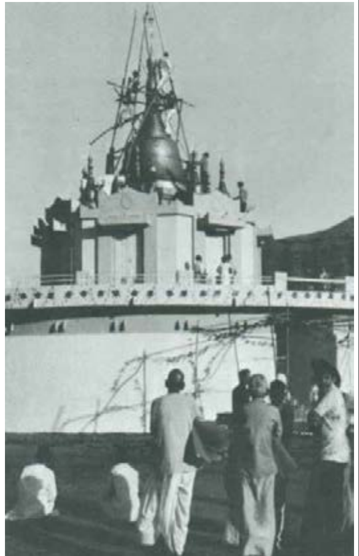
Students completing installation of metal umbrella, in preparation for the inauguration of the Pagoda (March 15, 1979).
